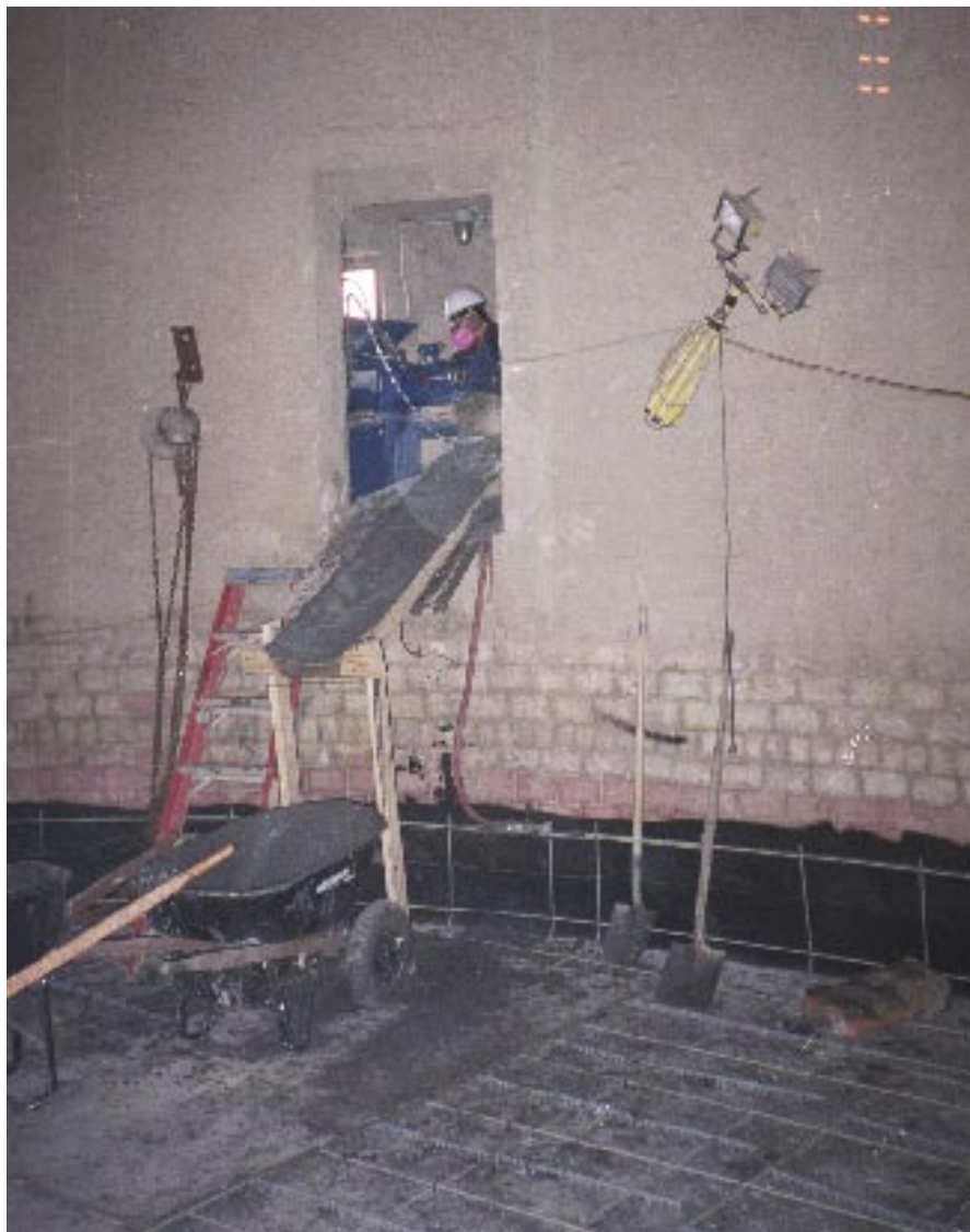
Application of polymer concrete to a brick chimney floor. The concrete was prepared in a continuous mixer and poured through the chute to the foundation below.
