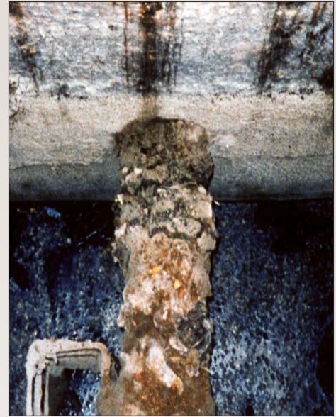
The Las Vegas project exhibited corrosion within the vapor zone, similar to this lift station in Louisiana.
