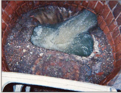
Las Vegas manholes exhibited deteriorated mortar joints and corrosion of concrete.
