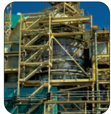
Exterior view of a protected scrubber module.
