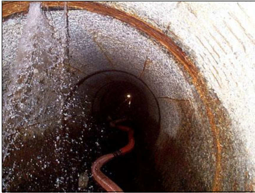
# 1 - Pipeline showing dramatic evidence of corrosion and water inflow.
