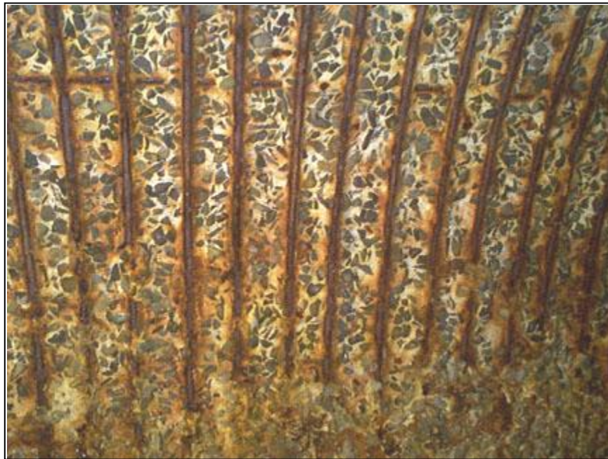
#2 – Exposed aggregate and corroded rebar illustrate the critical need for restoration.
