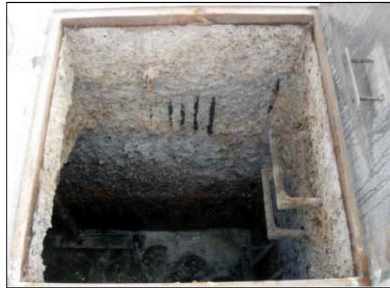
Severe corrosion in underground utility vault
