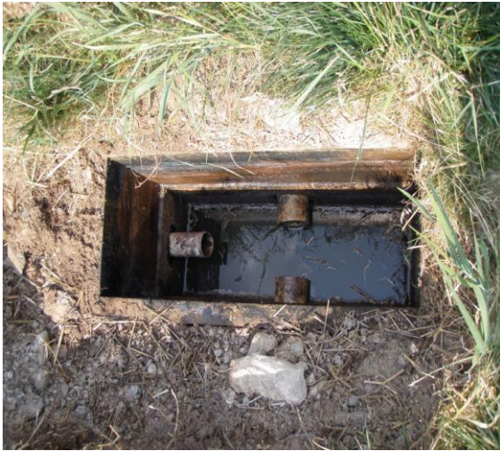
Concrete drainage vault before rehabilitation
