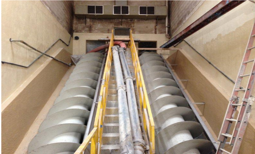
Sauereisen's SewerGard No. 210 protects concrete from abrasion & corrosion at the O.C.U.A – CPS-11 Lacy-Middle Branch Lift Station 490 U.S. Route 9
