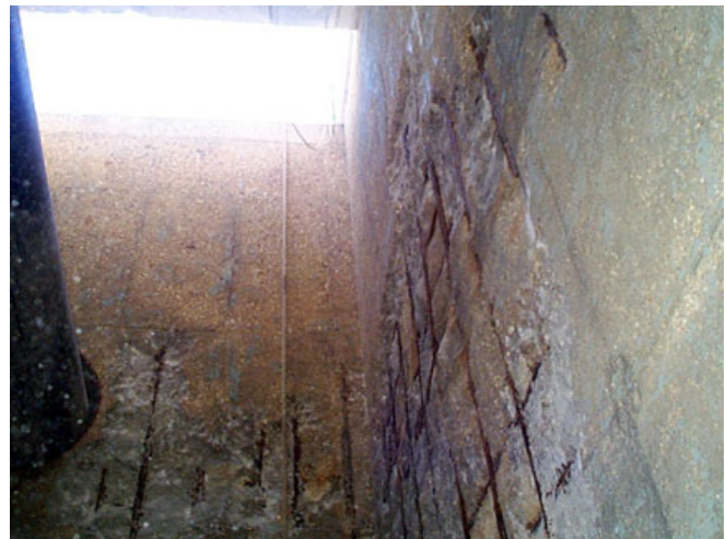
Severe degradation to pump station walls
