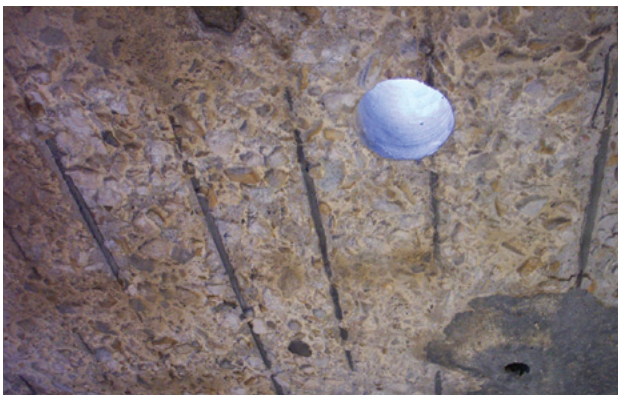
Concrete in wet-well deteriorated to reinforcement
