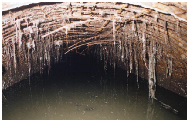
The crown section of this 14' tunnel experience severe degradation
