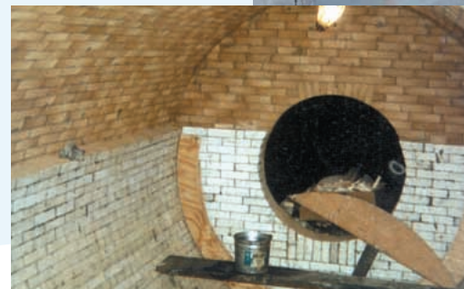
Brick and Sauereisen mortar provide longevity for this scrubber vessel within a sulfur recovery unit.
