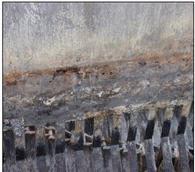
Figure 2 Stainless steel tank wall with holes resulting from MIC.
