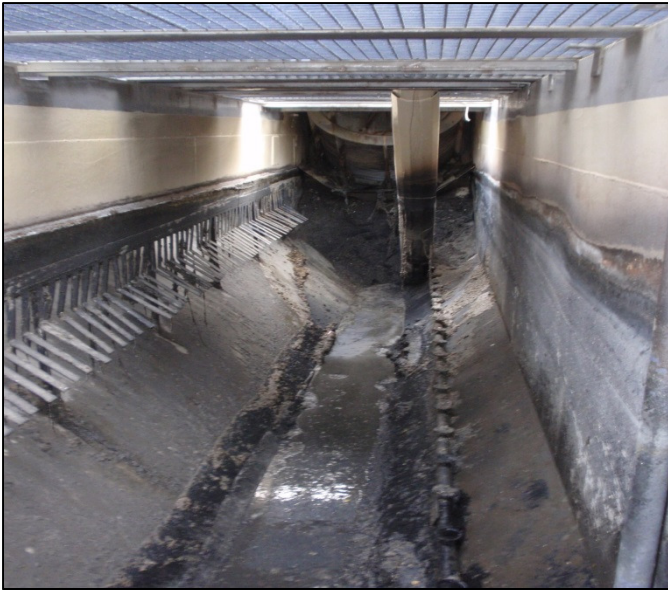
Figure 3 View looking down the tank after six months in service (tank cleaned).
