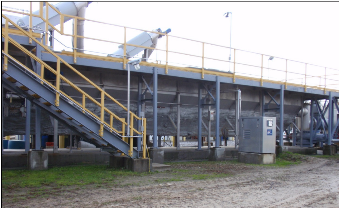
Figure 1 Above grade stainless steel headworks tank at Logan Township MUA
