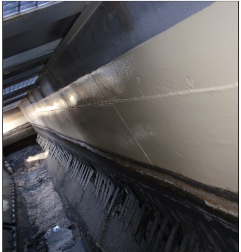
Figure 4 Coated stainless steel sidewall after six months in service (tank cleaned).
