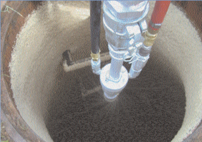
IPC Inc. used spin-casting equipment to apply Sauereisen Substrate Resurfacer F-121 to grout and repair manhole surfaces.
