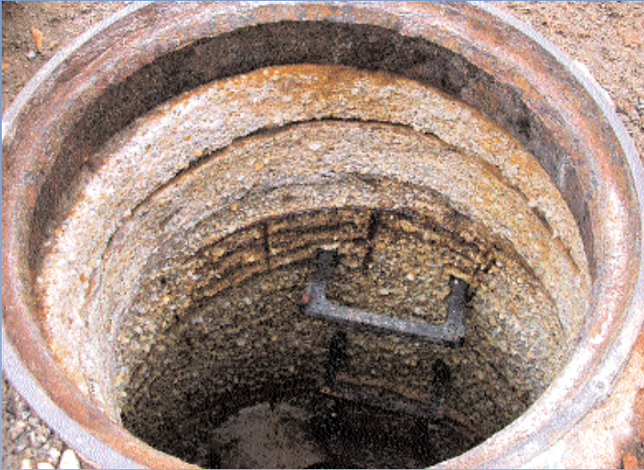
A highly corroded manhole before treatment in the City of Pace, Fla.'s preventative maintenance program was instituted.
