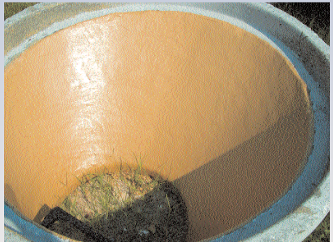
Manholes in the City of Pace, Fla., were coated with Sauereisen's SewerGard 210 epoxy.
