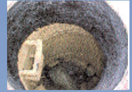
An after picture of one of the rehabbed manholes in the City of Pace, Fla.
