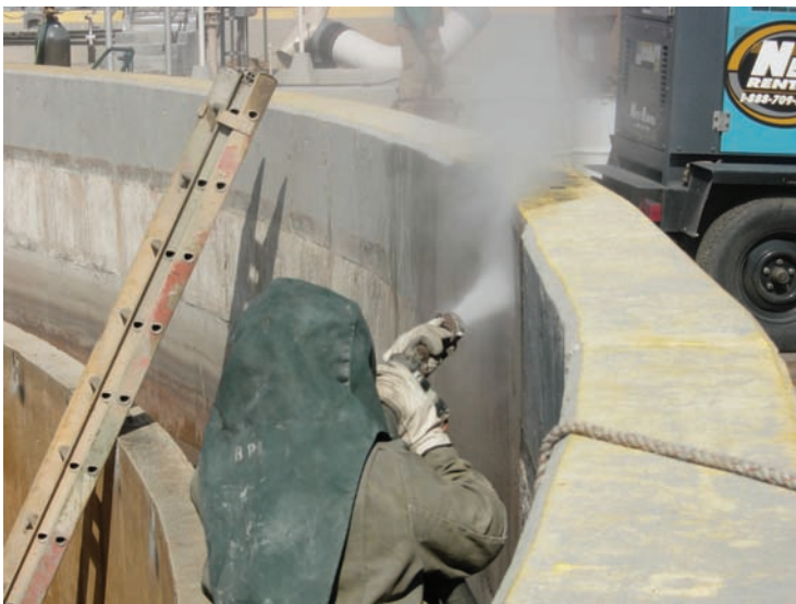
A combination of abrasive and high-pressure water was used to prepare the concrete.
