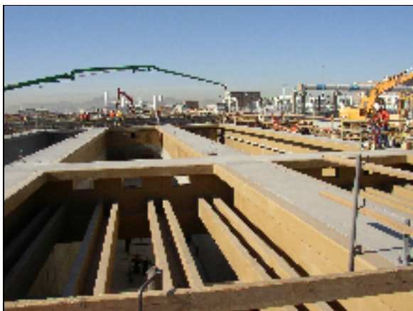
Coated grit chambers
