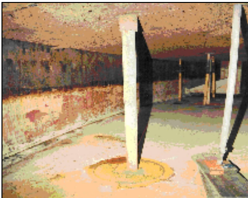
Corrosion on floors & walls
